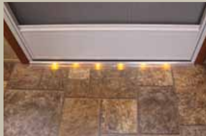
Amber threshold lighting at main entrance for added safety.
